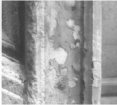
Figure 25. The clear coating applied to this limestone masonry has failed and is taking off some of the stone surface as it peels. Photo: Frances Gale.
