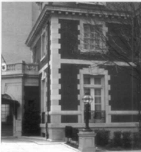
Figure 4. The foundation of this brick building is limestone, but the decorative trim above is architectural terra cotta intended to simulate stone.
