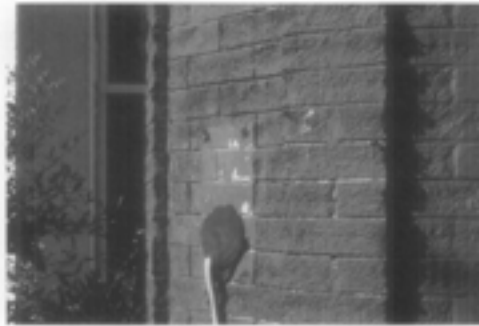
Figure 19. A comparison of undamaged bricks surrounding the electrical conduit with the rest of the brick facade emphasizes the severity of the erosion caused by sandblasting.
