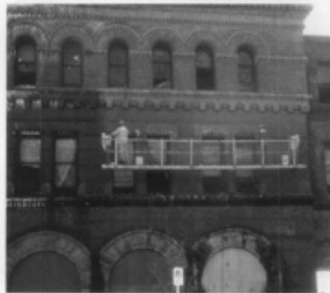
Figure 12. A mild acidic cleaning agent is being used to clean this heavily soiled brick and granite building. Additional applications of the cleaner and hand-scrubbing, and even poulticing, may be necessary to remove the dark stains on the granite arches below. Photo: Sharon C. Park, FAIA.
