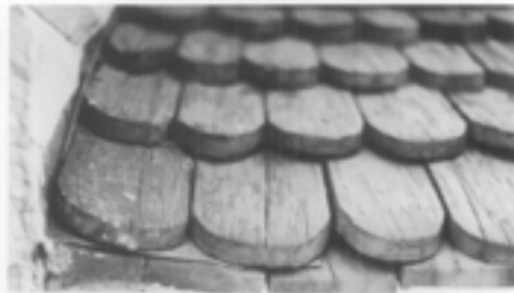
Replacement of particular historic details is important to the individual historic character of a roof, such as the treatment at the eaves of this rounded butt wood shingle roof. Also note that the surface of the roof was carefully sloped to drain water away from the side of the dormer. In the restoration, this function was augmented with the addition of carefully concealed modern metal flashing. (Mount Vernon, Virginia)
