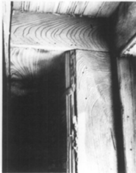
Abrasive Cleaning of Wood. This wooden windowsill, molding and paneling have been sandblasted to remove layers of paint in the rehabilitation of this commercial building. Not only is some paint still embedded in cracks and crevices of the woodwork, but more importantly, grit blasting has actually eroded the summer wood, in effect raising the grain, and resulting in a rough surface.
