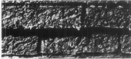
Hazards of Sandblasting and Surface Coating. In order to "protect" this heavily sandblasted brick, a clear surface coating or sealer was applied. Because the air temperature was too cold at the time of application, the sealer failed to dry properly, dripping in places, and giving the brick surface a cloudy appearance.
