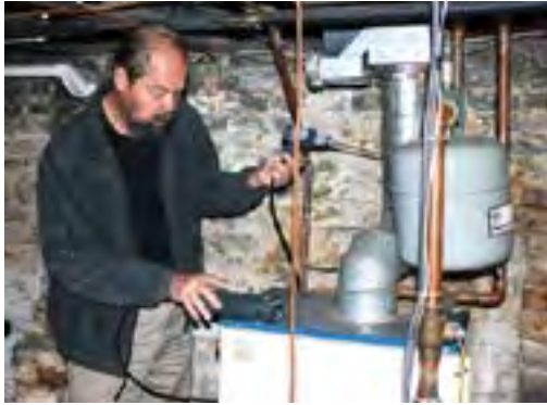
Fig. 9. An energy auditor tests the efficiency of a boiler.
