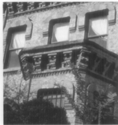
Figure 15. The whitish deposits left on the brick by a chemical paint remover may have resulted from inadequate rinsing or from the chemical being left on the surface too long and may be impossible to remove.
