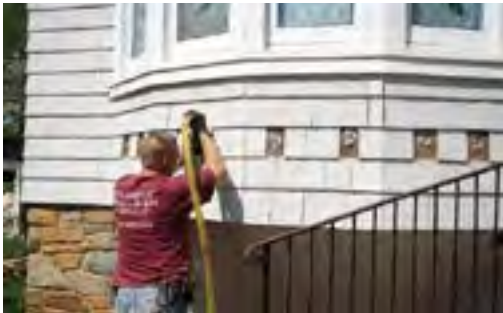
Fig. 18. Dense-packed cellulose insulation is being blown in through holes drilled in the sheathing. Once the operation has been completed, the shingles will be reinstalled. Photo: Edward Minch.
