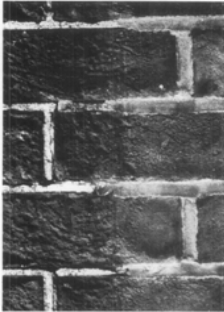
Abrasively Cleaned vs. Untouched Brick. Two brick rowhouses with a common facade provide an excellent point of comparison when only one of the houses has been sandblasted. It is clear that abrasive blasting, by removing the outer surface, has left the brickwork on the left rough and pitted, while that on the right still exhibits an undamaged and relatively smooth surface. Note that the abrasive cleaning has also removed a considerable portion of the mortar from the joints of the brick on the left side, which will require repointing.
