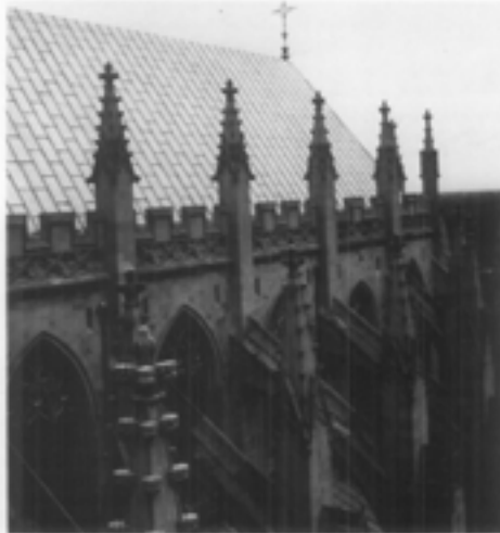
Good design and quality materials for the roof surface, fastenings, and flashing minimize roofing failures. This is essential on roofs such as on the National Cathedral where a thorough maintenance inspection and minor repairs cannot be done easily without special scaffolding. However, the success of the roof on any structure depends on frequent cleaning and repair of the gutter system. (Washington, D.C., photo courtesy of John Burns, A.I.A.)
