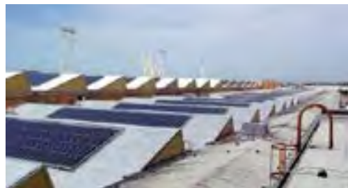
Fig. 23. Solar collectors installed in a compatible manner on low sloping sawtooth monitors. Top Photo: Neil Mishalov, Berkeley, CA.
