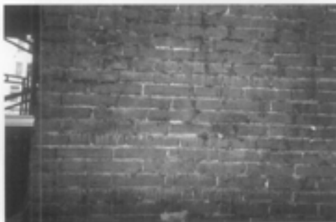
Figure 13. Sometimes it may be preferable to paint over a thick asphaltic coating rather than try to remove it, because it can be difficult to remove completely. However, in this case, many layers of asphaltic coating were removed through multiple applications of a heavy duty chemical cleaner. Each application of the cleaner was left to dwell following the manufacturer's recommendations, and then rinsed thoroughly. (As much as possible of the asphalt was first removed with wooden scrapers.) Although not all the asphalt was removed, this was determined to be an acceptable level of cleanliness for the project.
