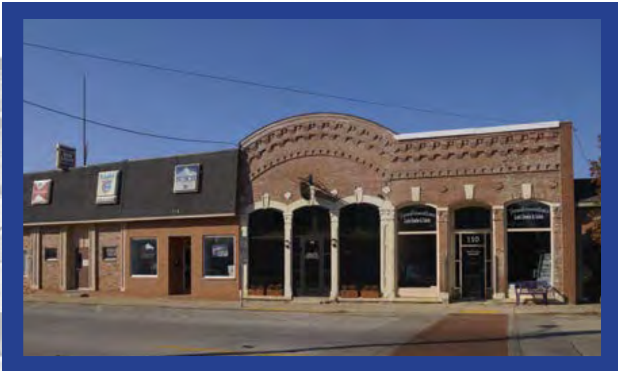
The removal of the modern storefront to reveal the historic brickwork during the rehabilitation of this west facade reveals important unique details of the historic facade.
